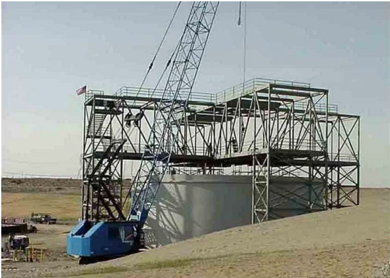
The Hanford Site's Cold Test Facility went into service in summer 2002 and features a full-scale mock-up of a single-shell waste storage tank.
