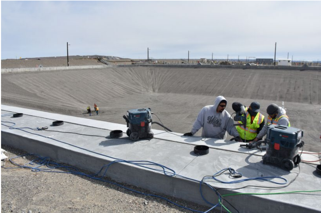
Elite Construction & Development assisted in constructing a liquid retention basin, one of many significant upgrades required to support the Direct-Feed Low-Activity Waste Program to treat tank waste at the Hanford Site.
