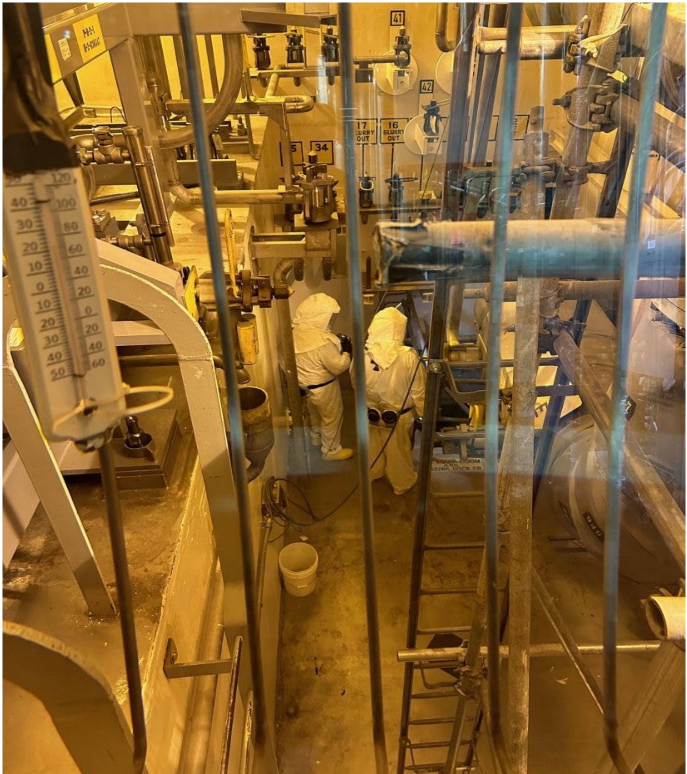
Crews conduct an initial inspection inside the Hanford Site's 242-A Evaporator to prepare for system startup.
