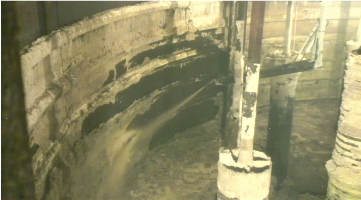
The water stream from one of three sluicers installed in AX-101 on the Hanford Site is used to remove waste from tank walls during retrieval operations.
